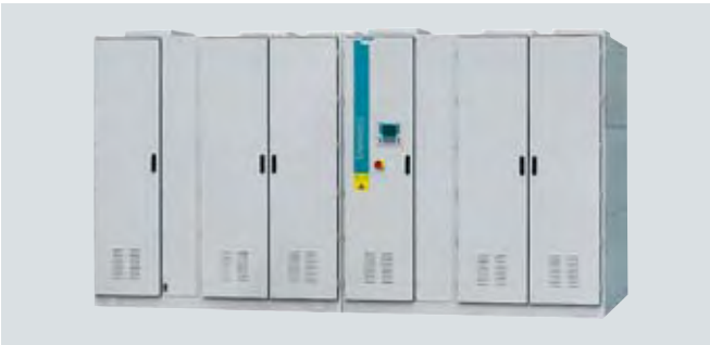
The drive solution for single-motor and multi-motor drives in the medium-voltage range
